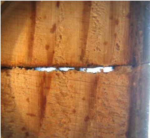
Fig. 7: Crack in Glue Line and Seal
