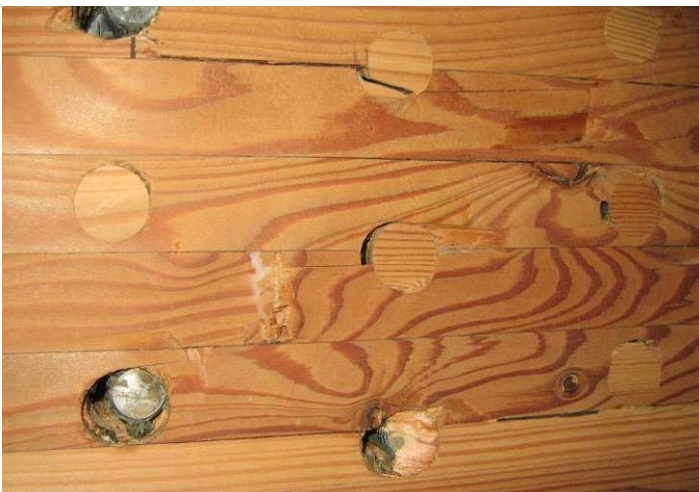
Fig. 3: Shear and Tension Cracks at the main joint
