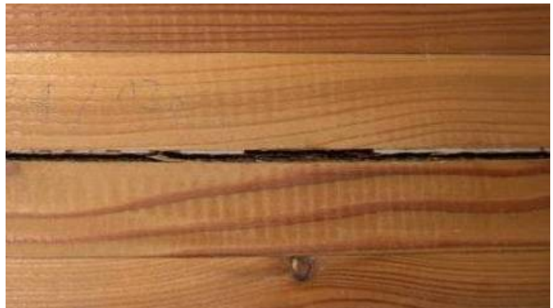
Fig. 8: Crack in formerly sealed Glue Line
